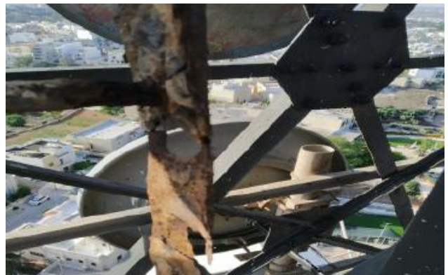
Damage on the Transmission Tower
