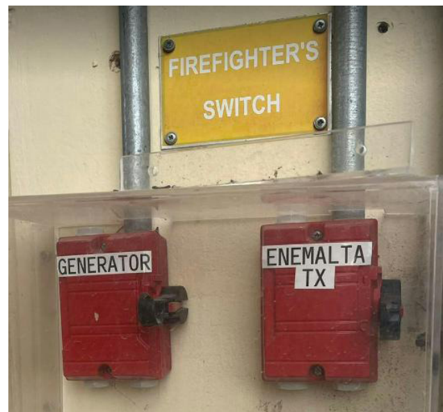
Fireman Emergency Switches
